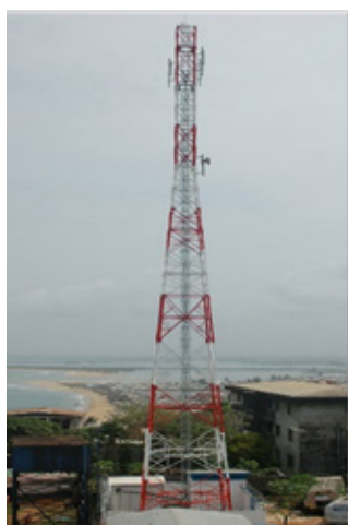
Menara kekisi berkaki empat (four-legged lattice tower)
